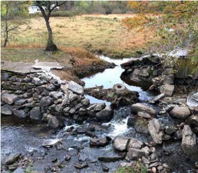
In 2018 the dam failed and created an impasse for fish. Aspetuck Land Trust applied for funding from the EPA to remove the dam to create a fish passage.
