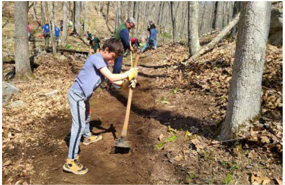
Benching a new trail in Trout Brook Valley in orange trail reroute.
