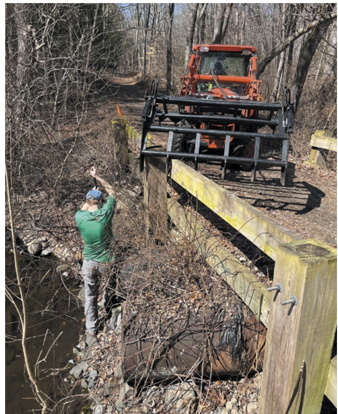
ALT staff repairing the bridge at the Hawley's Brook fish ladder in Trout Brook Valley.
